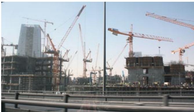
Student delegates viewed firsthand some of the numerous immense construction projects underway in Saudi Arabia, the one pictured here being the site of the Riyadh-based future HRH Princess Noura Bint Abdulrahman University, which, upon completion, will be the world's largest all-women's institution of higher education.
